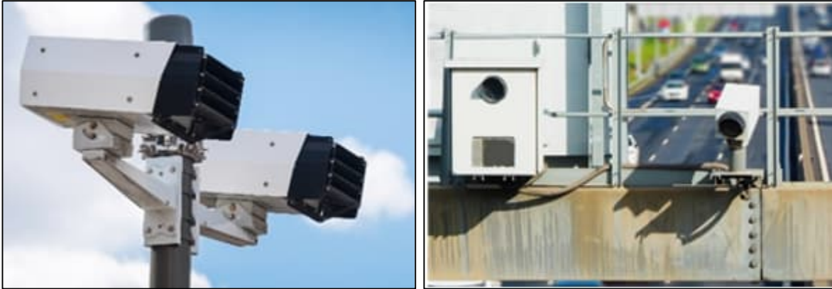
Figure 5-12. CCTV Camera and Radar Detection for TPAS
