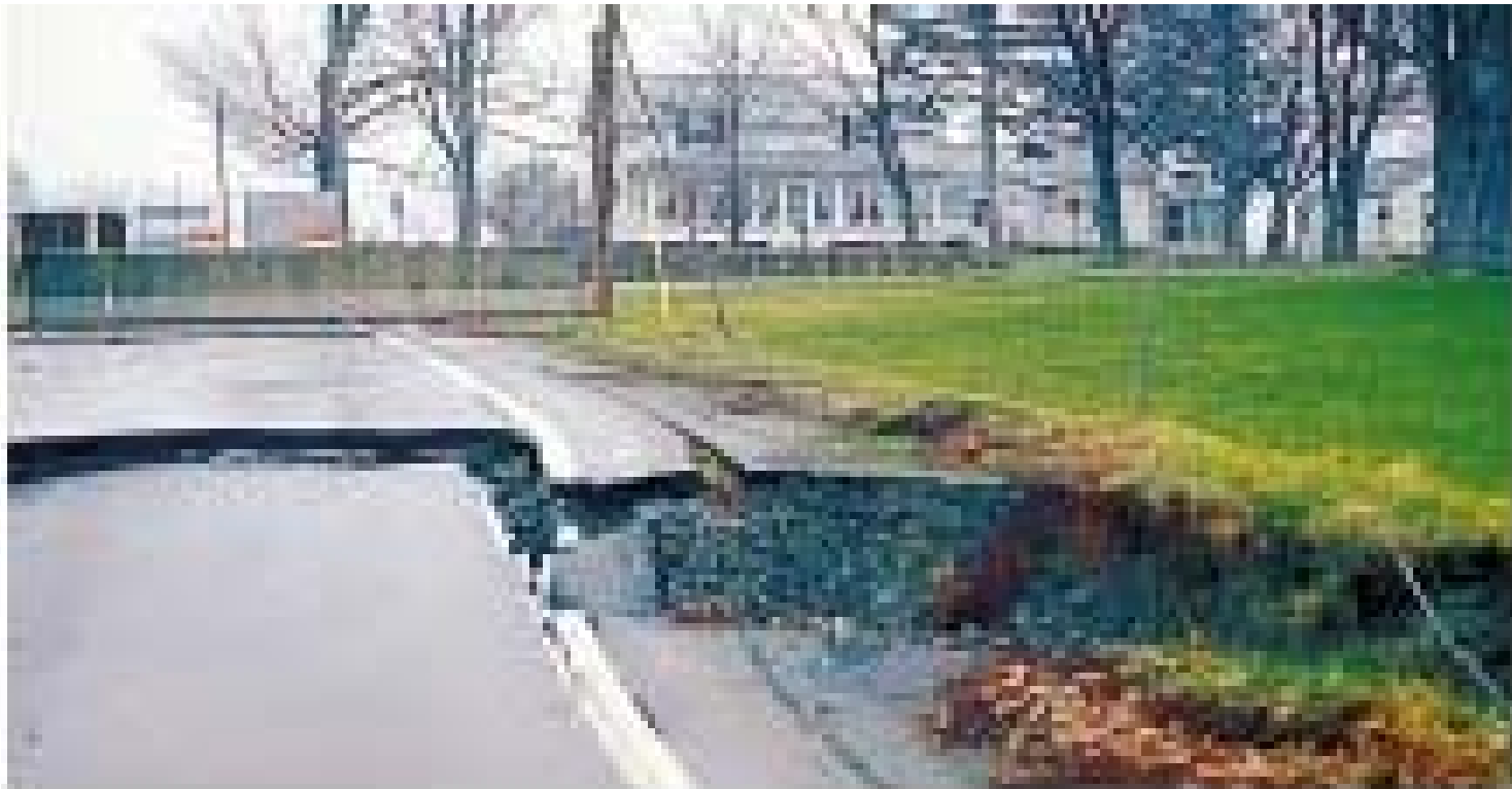
A roadbed fractured above the mine collapse area.
