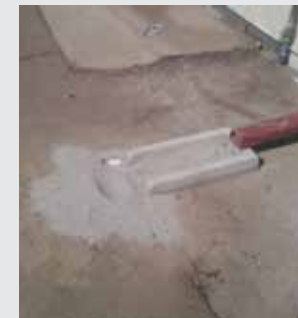
This image shows aftermath of hail damage to shingles of the Traffic Signals Sign & Striping building. Rain washed the pulverized shingle material down the spout.
