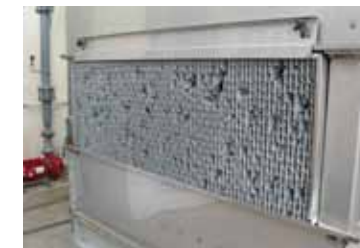
The recent hail storm damaged one of ADOT’s air cooling unit
