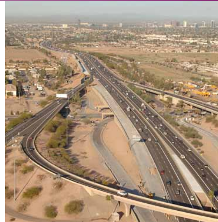
On the Loop 202 (Red Mountain Freeway) looking westward during construction: The McDowell Road off-ramp lies in the foreground with downtown Phoenix in the background.
