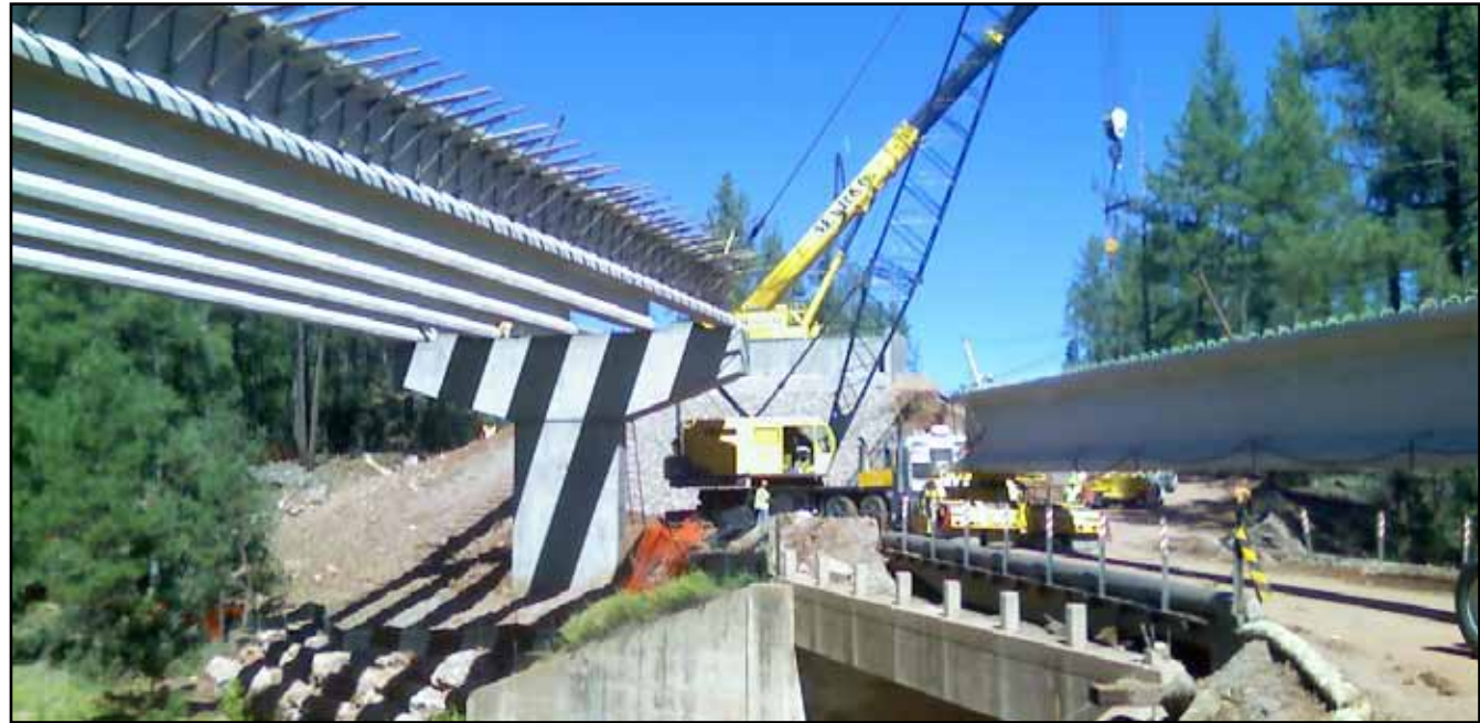
Bridging past and present – Jon Lenzmeier, a tech 1 from Payson Construction, sent us this photo showing the contrast between the old and new bridges over the Thompson Draw Wash on State Route 260, about 11 miles east of Payson in an area called Little Green Valley. A two-lane, undivided bridge was built in 1962. In 2004, it was replaced by a newer bridge that currently handles two-way traffic. That traffic will switch to the newest bridge (in photo) later this month, clearing the way for construction on the eastbound side of 260. When the entire project wraps up next summer, the newest bridge will carry westbound traffic, while the 2004-built bridge will carry eastbound traffic. The bridge construction is part of a larger project to widen 260 from two to four lanes. "It [the photo] really shows the magnitude of the expansion that is being done with the new westbound-only bridge being constructed," Lenzmeier wrote in an email.
