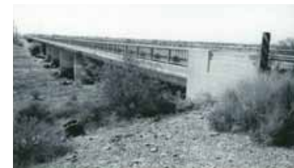
The Arizona Highway Department built this bridge in the 1950s to replace the 1910 bridge.
