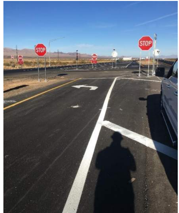
US 93 at Pierce Ferry Road. In Fall 2020, ADOT completed a project to modify the northbound and southbound US 93 left-turn lanes at the intersection. The US 93 at Pierce Ferry Road Feasibility Study evaluates grade-separation alternatives.
