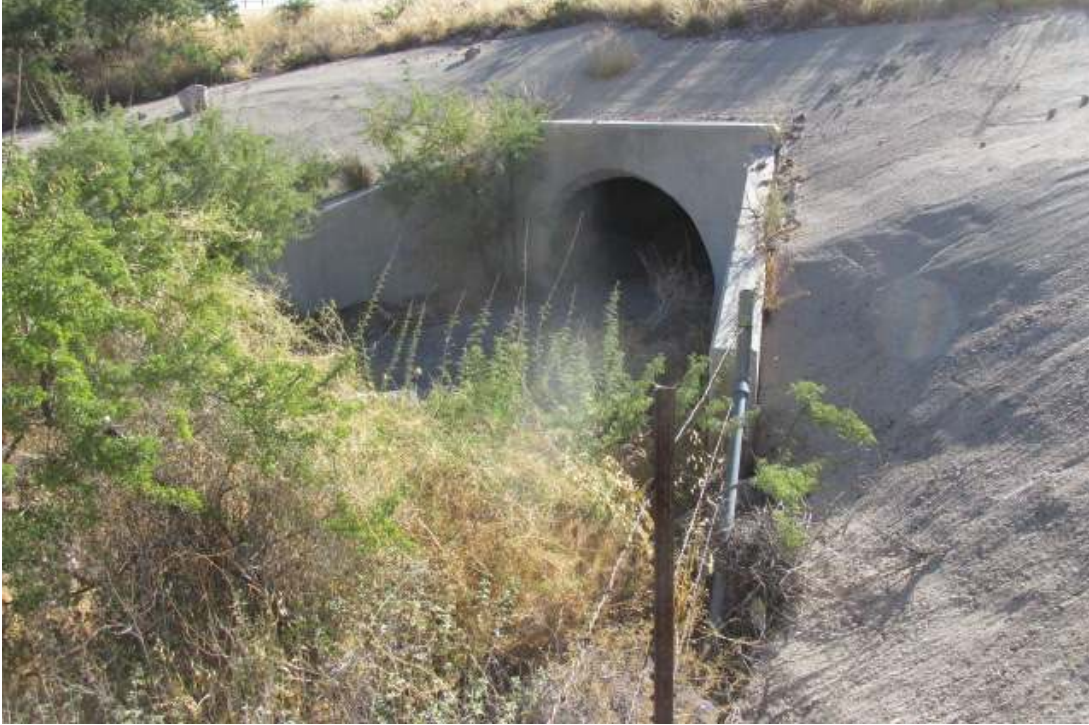
Photograph 9. View northeast of the I-40 reinforced corrugated metal pipe culvert (RCMP), near MP 48.3. Typical of the concrete drainage within the Study Area.
