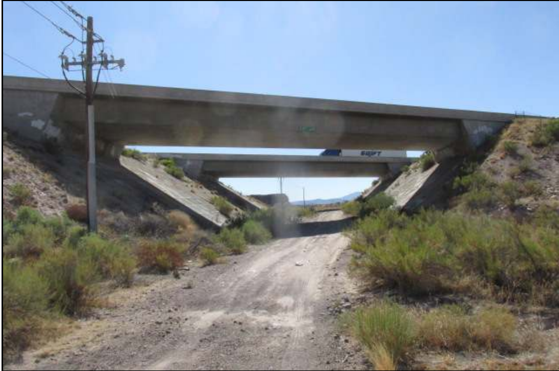
Photograph 11. View south of White Cliff Road OPs, I-40 at MP 50.09. Photograph date: October 1, 2019.
