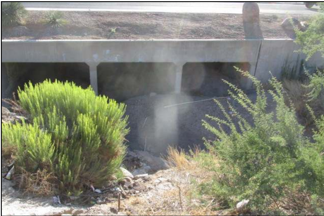
Photograph 12. View southwest of US 93 reinforced concrete box culvert (RCB) near MP 70.3. Photograph date: October 1, 2019.
