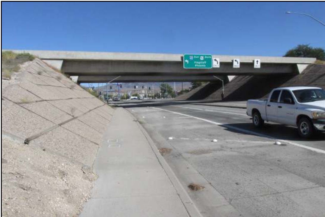
Photograph 10. View east of the West Kingman traffic interchange (TI) overpass (OP) eastbound (EB), I-40 at MP 48.4.
