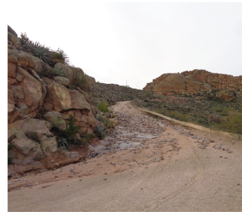
Narrow roadway, eroded surface
