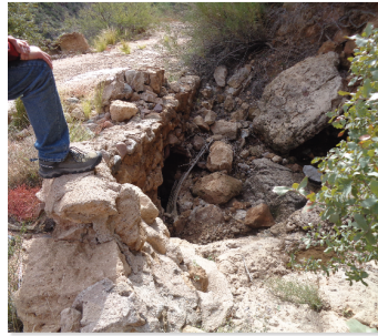
Drainage and erosion
