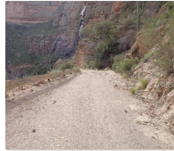
Guardrail is damaged and in poor condition
