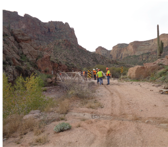
Bridge rehabilitation/ repairs are needed
