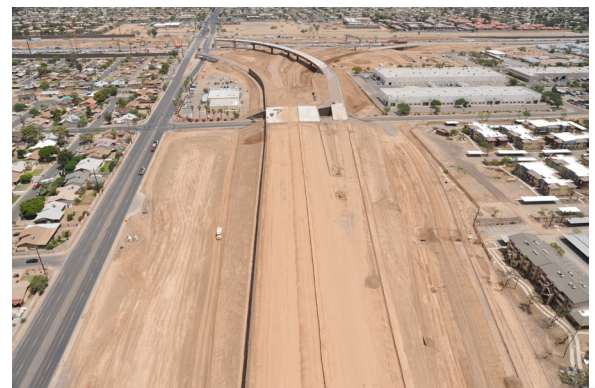
Aerial view of 59th Avenue south of Roosevelt Street prior to frontage road construction
