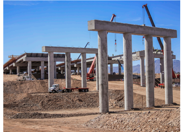
Constructing the two half-mile long Salt River bridges (Photo courtesy of ADOT)
