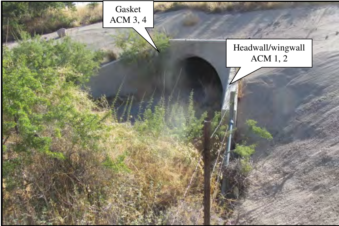
Photograph 1. View northeast of reinforced corrugated metal pipe (RCMP) along Interstate 40 (I-40), near milepost (MP) 48.3. Photograph date: October 2, 2019.
