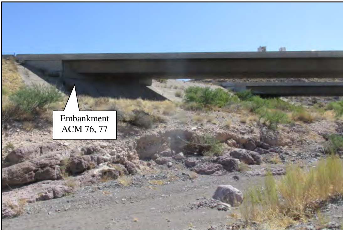
Photograph 16. View of the Clack Canyon Wash OP WB embankment slope. Photograph date: October 1, 2019.
