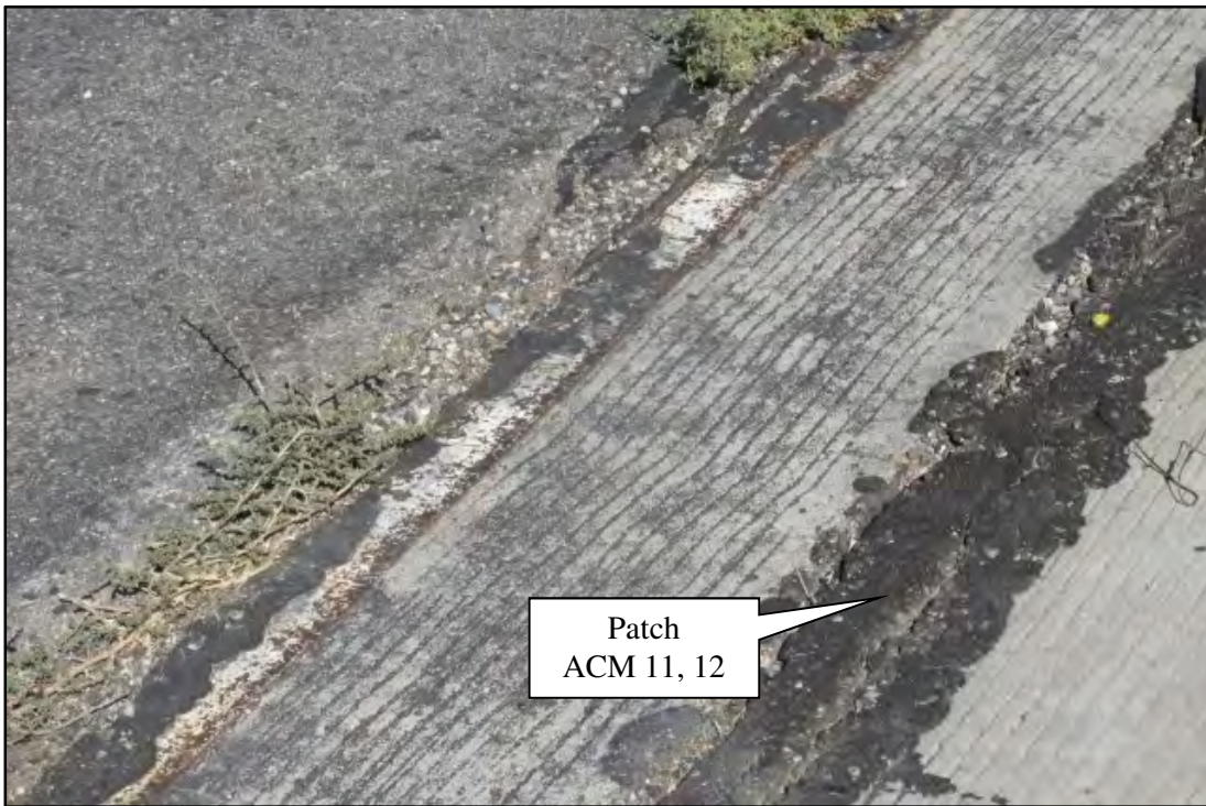
Photograph 4. Detail view of the West Kingman TI OP WB expansion joint patch. Photograph date: October 1, 2019.
