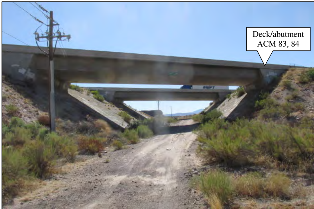
Photograph 22. View south of the White Cliff Road OP WB Structure #1840, MP 50.09 (foreground) and White Cliff Road OP EB Structure #1839, MP 50.09 (background). Photograph date: October 1, 2019.
