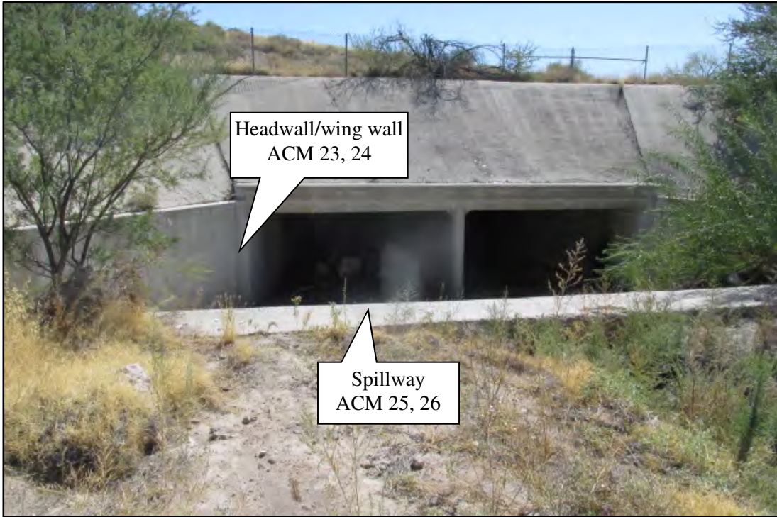
Photograph 13. Detail view of the West Kingman TI WB on-ramp reinforced concrete box culvert (RCB) and spillway. Photograph date: October 2, 2019.
