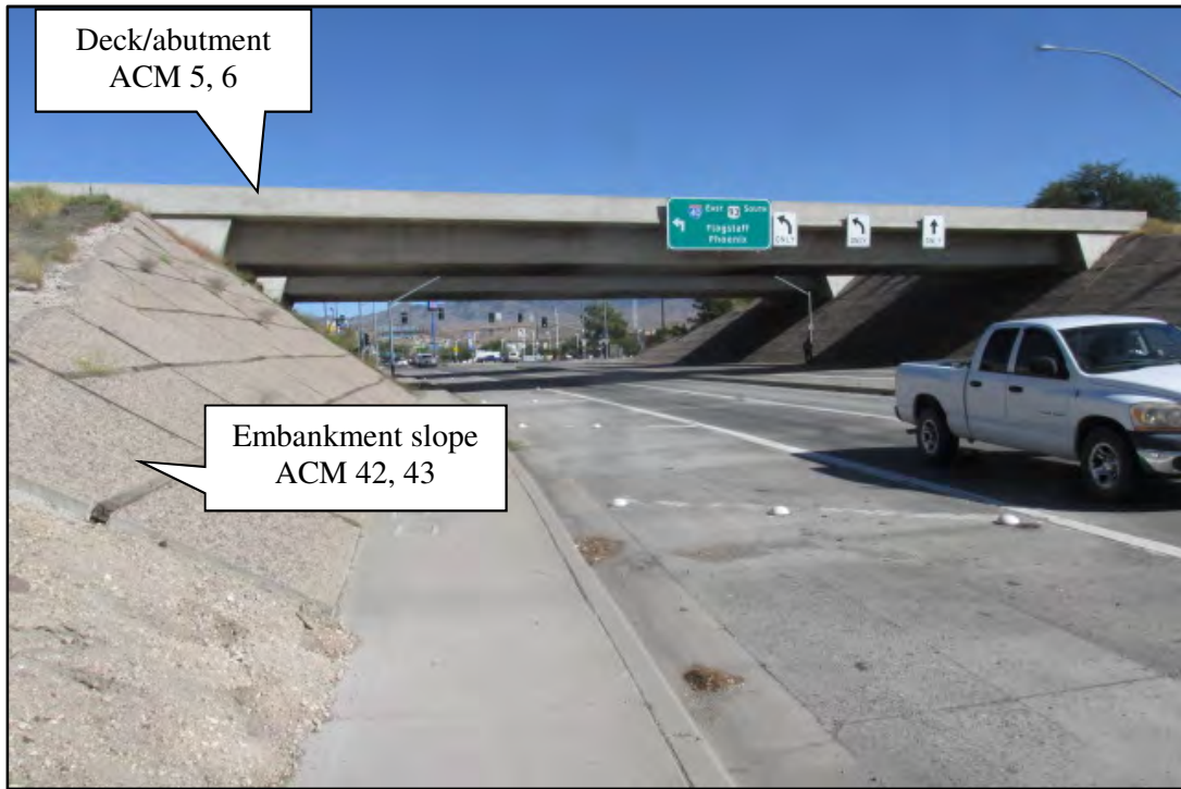
Photograph 2. View east of West Kingman traffic interchange (TI) overpass (OP) westbound (WB), Structure #1836, MP 48.84. Photograph date: October 1, 2019.
