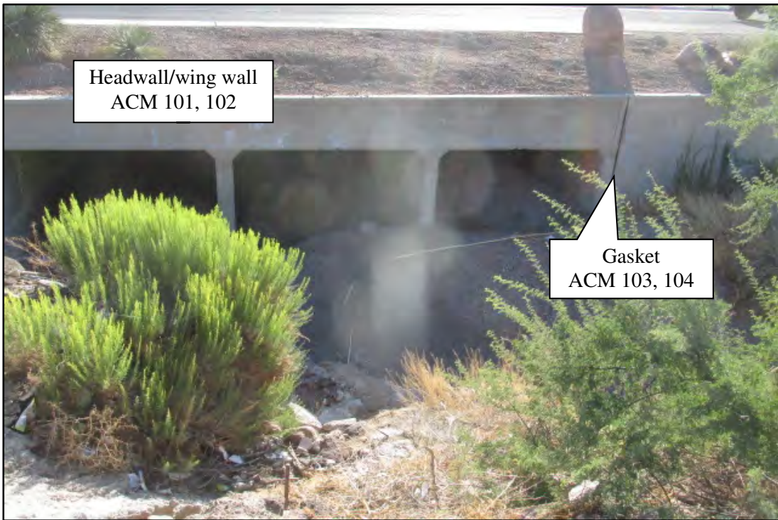
Photograph 26. View northeast of RCB under US Highway 93 (US 93), near MP 70.3. Photograph date: October 1, 2019.
