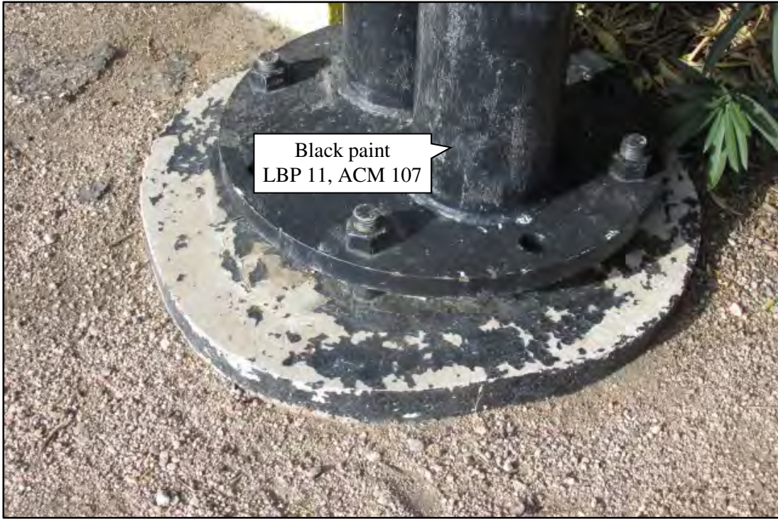
Photograph 29. Close-up view of black sign pole paint along US 93, near MP 70.3. Photograph date: October 16, 2019.
