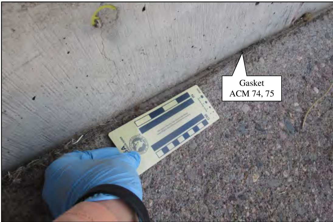
Photograph 18. View of the Clack Canyon Wash OP WB dado/embankment slope gasket. Photograph date: October 1, 2019.
