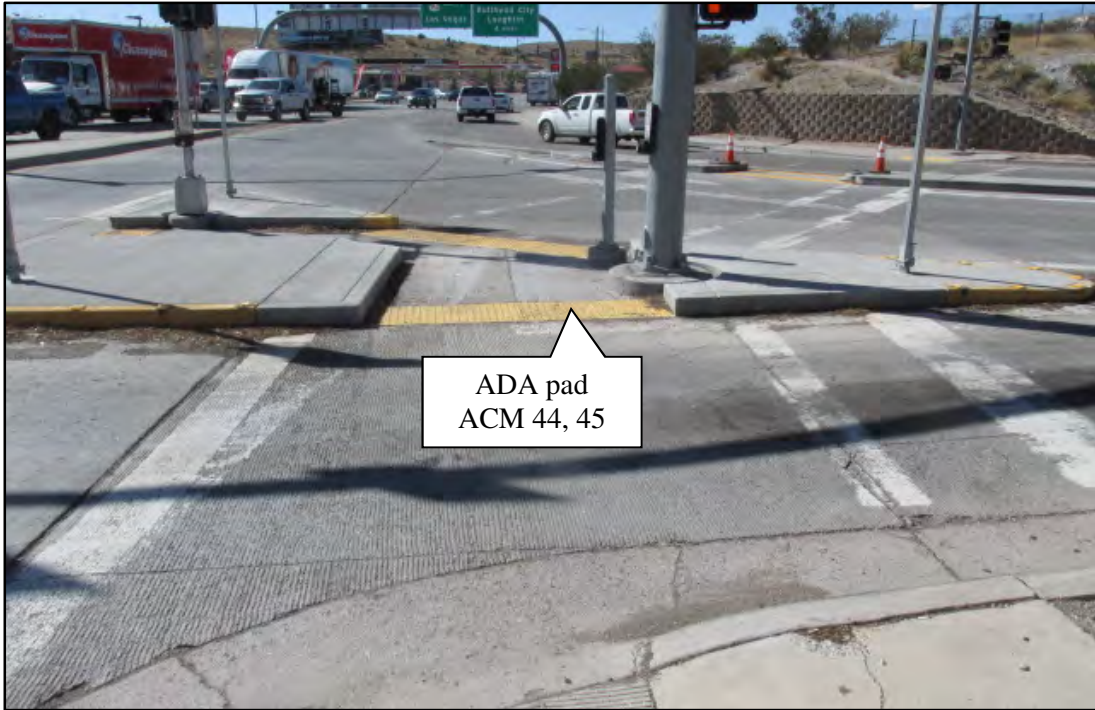
Photograph 5. View south of the West Kingman TI eastbound (EB)/WB Americans with Disabilities Act (ADA) yellow fiberglass pad. Photograph date: October 1, 2019.
