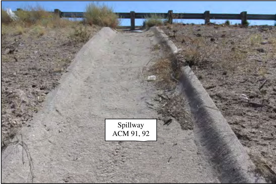
Photograph 25. View of the White Cliff Road OP WB spillway. Photograph date: October 1, 2019.
