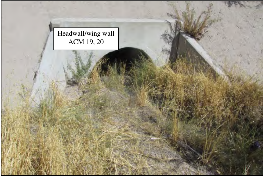
Photograph 11. Detail view of the West Kingman TI WB on-ramp SWC RCMP. Photograph date: October 2, 2019.
