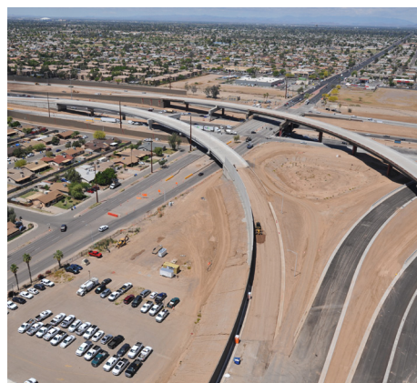
AFTER: Looking northwest toward I-10 Papago Freeway interchange at 59th Avenue April 2019
