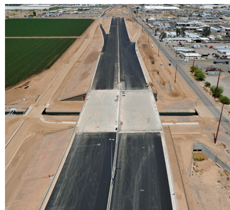
AFTER: Looking north toward Lower Buckeye Road at Roosevelt Irrigation District (RID) canal April 2019
